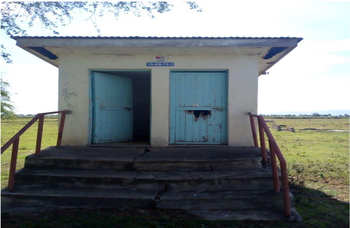
Plate 4. 7: A raised pit latrine whose floor suffered damages from floods was constructed by JICA at Magina in 2010 (Source: Author May, 2019)
