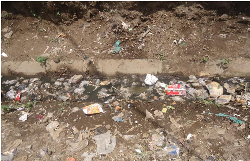
Plate 7: Photo Showing Blocked storm drainage
