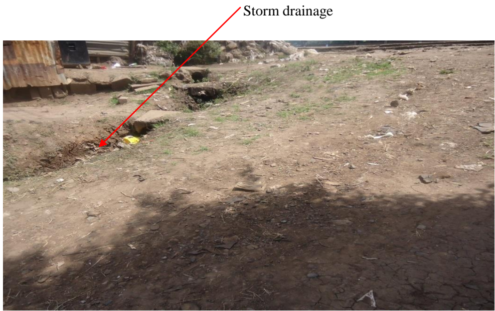
Plate 3: Photo showing dilapidated state of storm drainage
