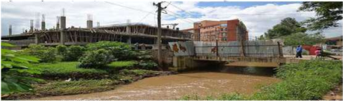
Two buildings are under construction on the banks of River Ngong near T-Mall on Mbagati Road (Photo: Courtesy)
