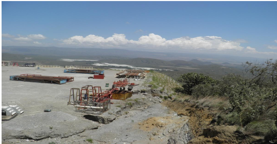
Plate 4.5: Disturbed site for well drilling in Hell's Gate National Park
