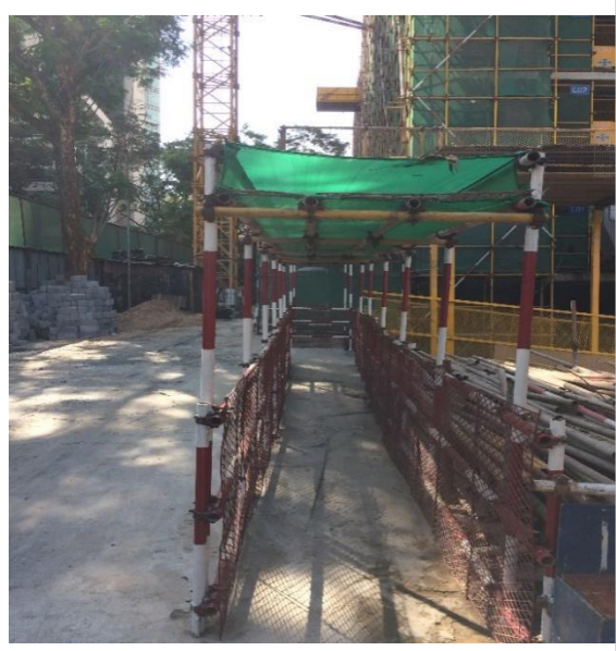
Walk ways well covered to protect against the falling object
