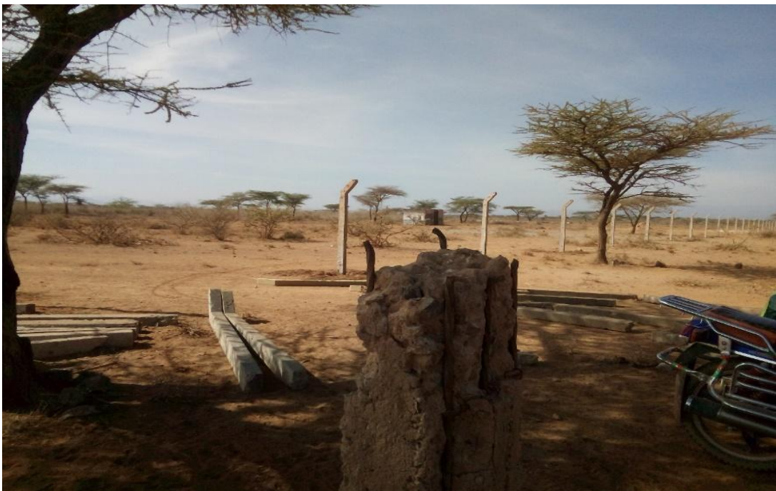
Figure 4.13: Erection of permanent fences to affirm claims to land and with anticipation to develop permanent structures
