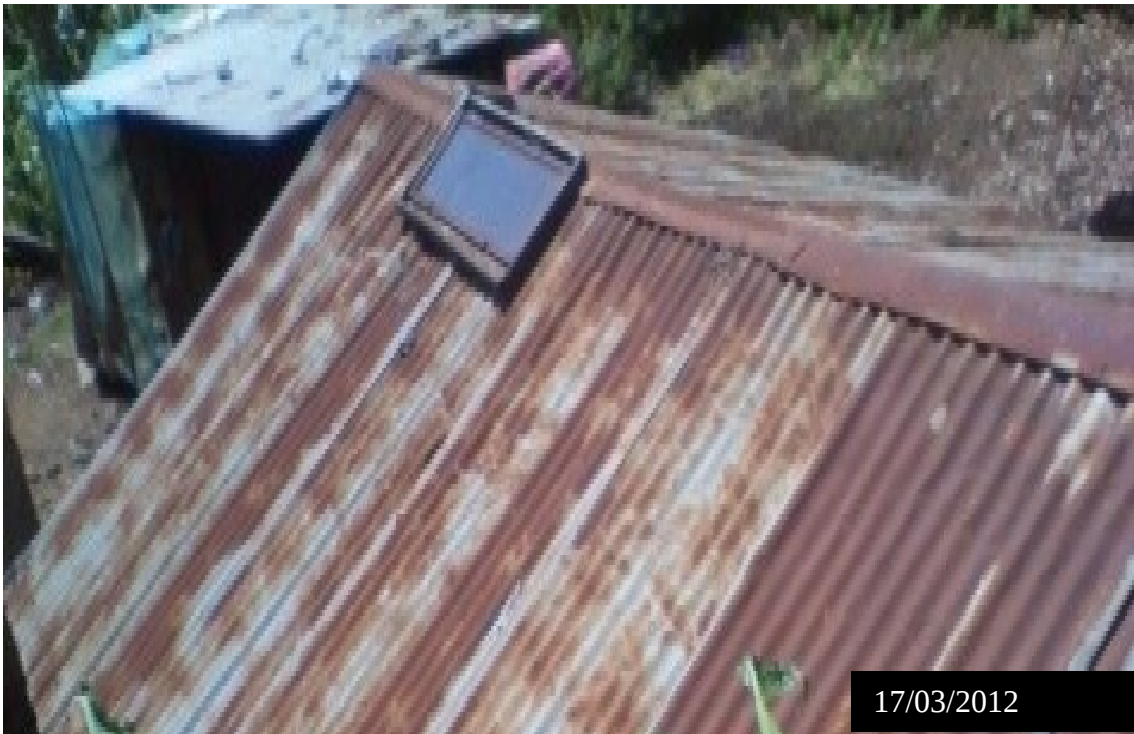
Plate 4.3 PV solar home system mounted on rooftop in Kauthini Source: Author (2012)
