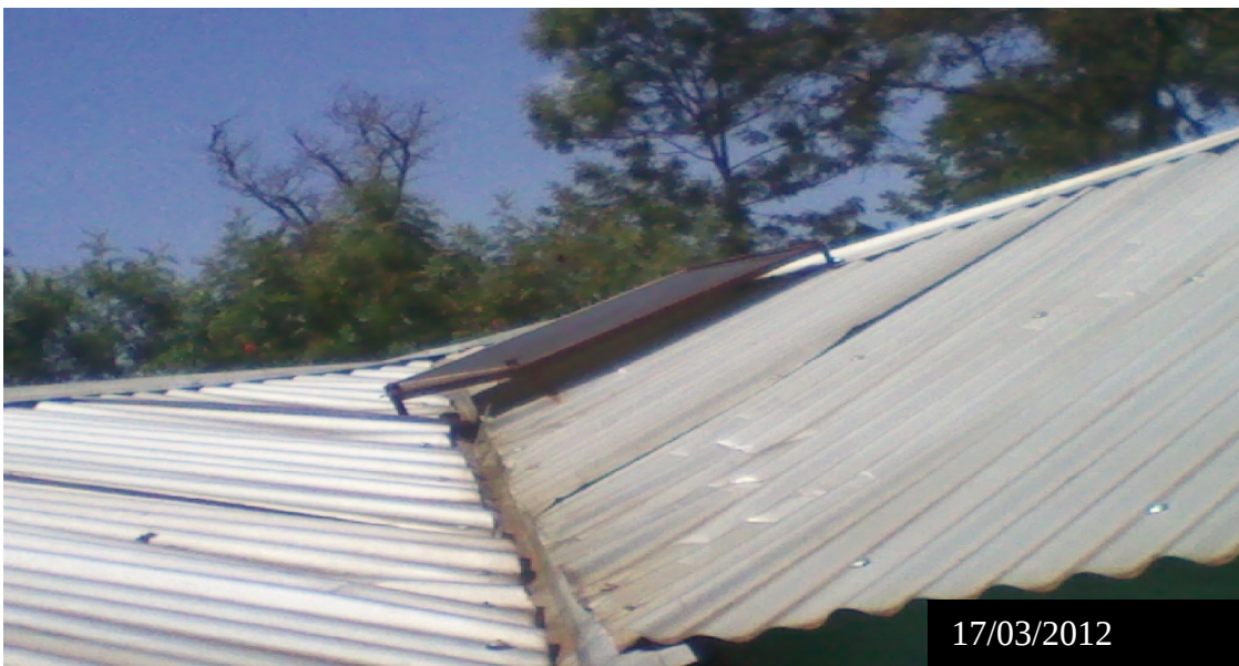
Plate 4.2 PV solar home system mountd on rooftop in Murunguma
