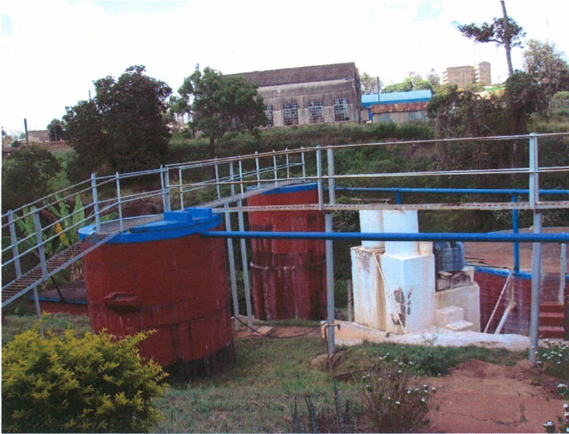
Plate 5.2: Ruiru water supply treatment facility
