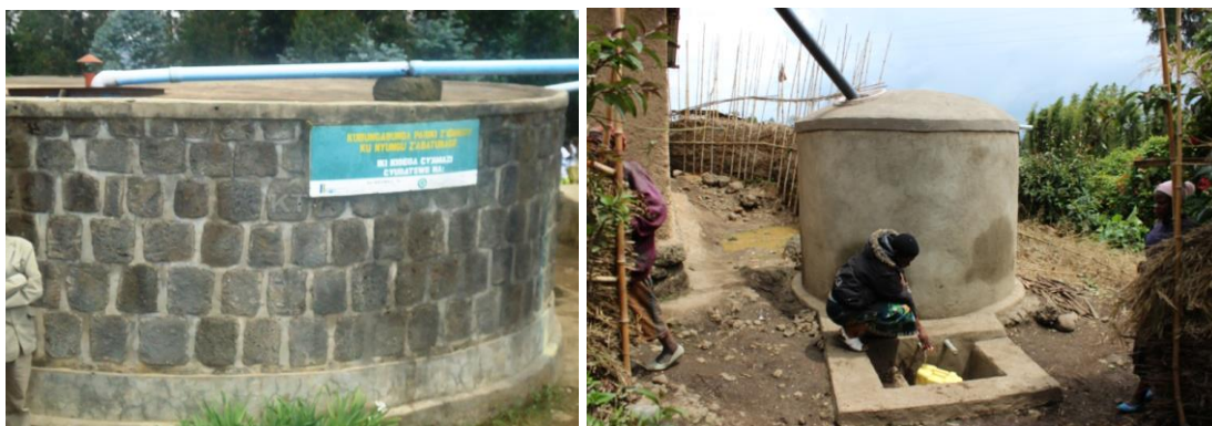
Plate 4.1: Water tanks constructed for households around VNP
