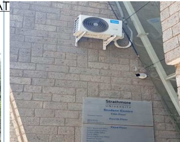
Image of air conditioner on exterior wall Source: James K. (2025)
