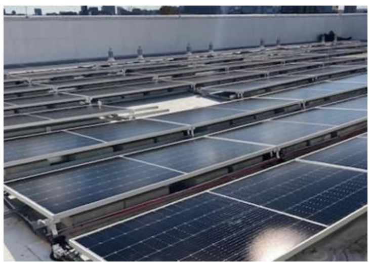
Figure Solar panels on building W46 Source: https://sustainability.mit.edu/
