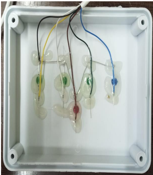
A picture showing the wiring of system state LEDs
