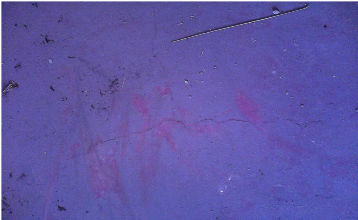
Plate 2-5: Developing cracks on the floor of a newly built house
