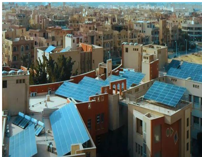
Solar panel layout on rooftop of Hayah International Academy Source: Presentation by Cairo Solar on how solar helped Hayah international academy save electricity. https://youtu.be/Wf24ZHvZGyQ?si=oMqP_gHWs26AGjs0
