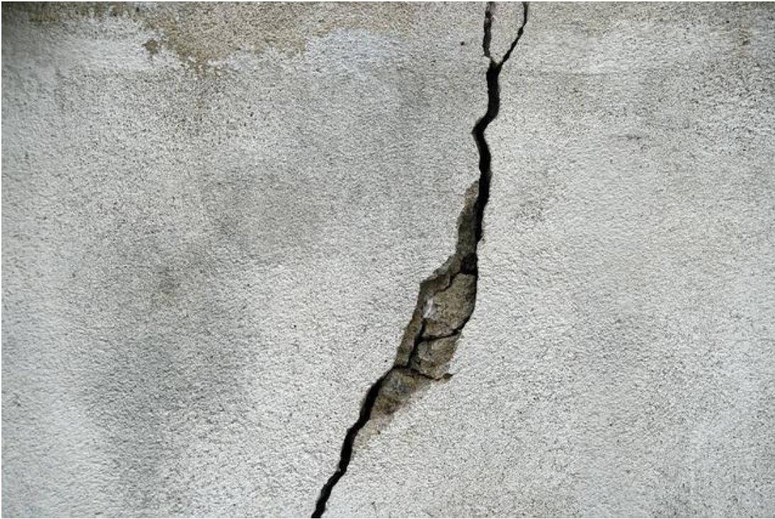
Plate 4.2: Cracked House Walls
