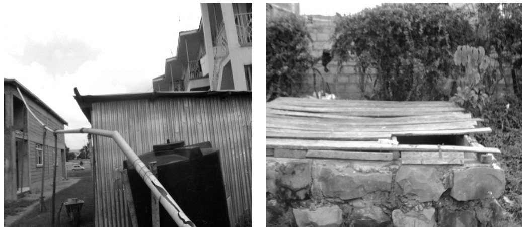
Plate 2: Improved mechanism for rainwater harvesting by a church in Embakasi; from left is the piping system followed by an underground concrete storage reservoir.
