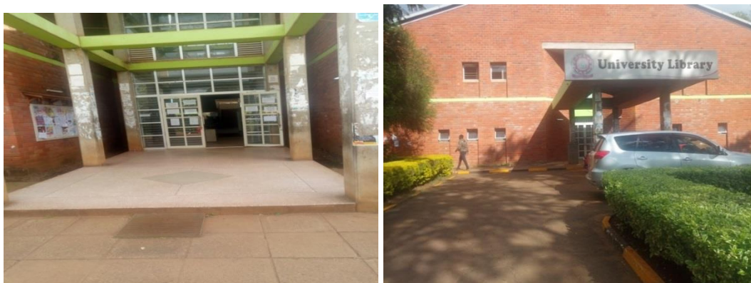
Figure 4.13 JKUAT – Disability Unfriendly buildings – Library entrances – No ramps nor climbing lane
