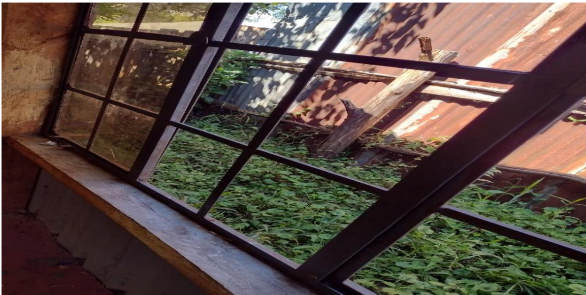
Figure 4.8: An example of an unsafe window without window panes.
