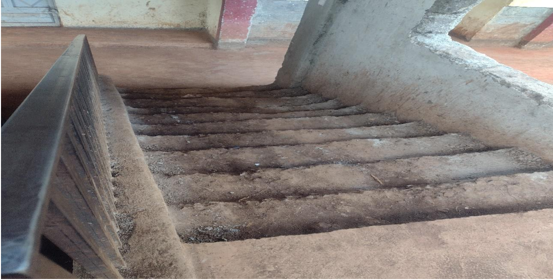
Figure 4.9: An example of an inappropriately Constructed staircase
