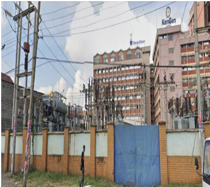
KPLC Workstation Source: author, 2024
