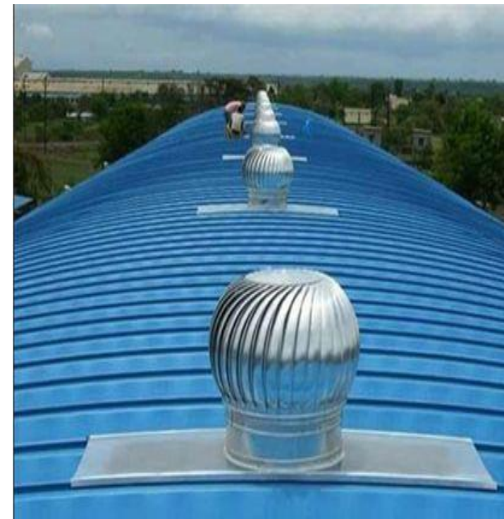
Rooftop turbines Source: author, 2024
