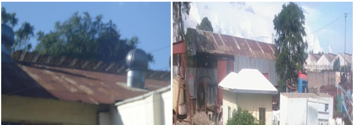
Plate 5-6: corroded roof tops in sections of industrial area
