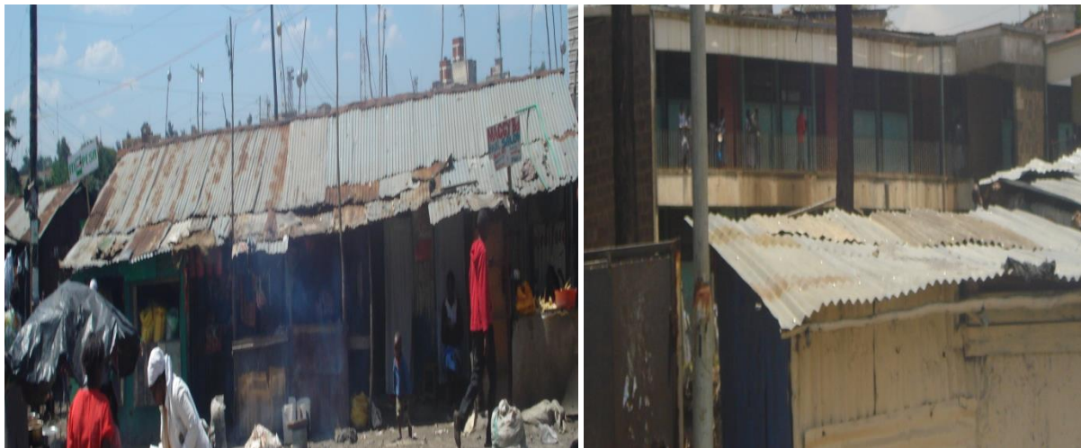
Plate 5-1: poor housing conditions; made of corrugated iron sheets
