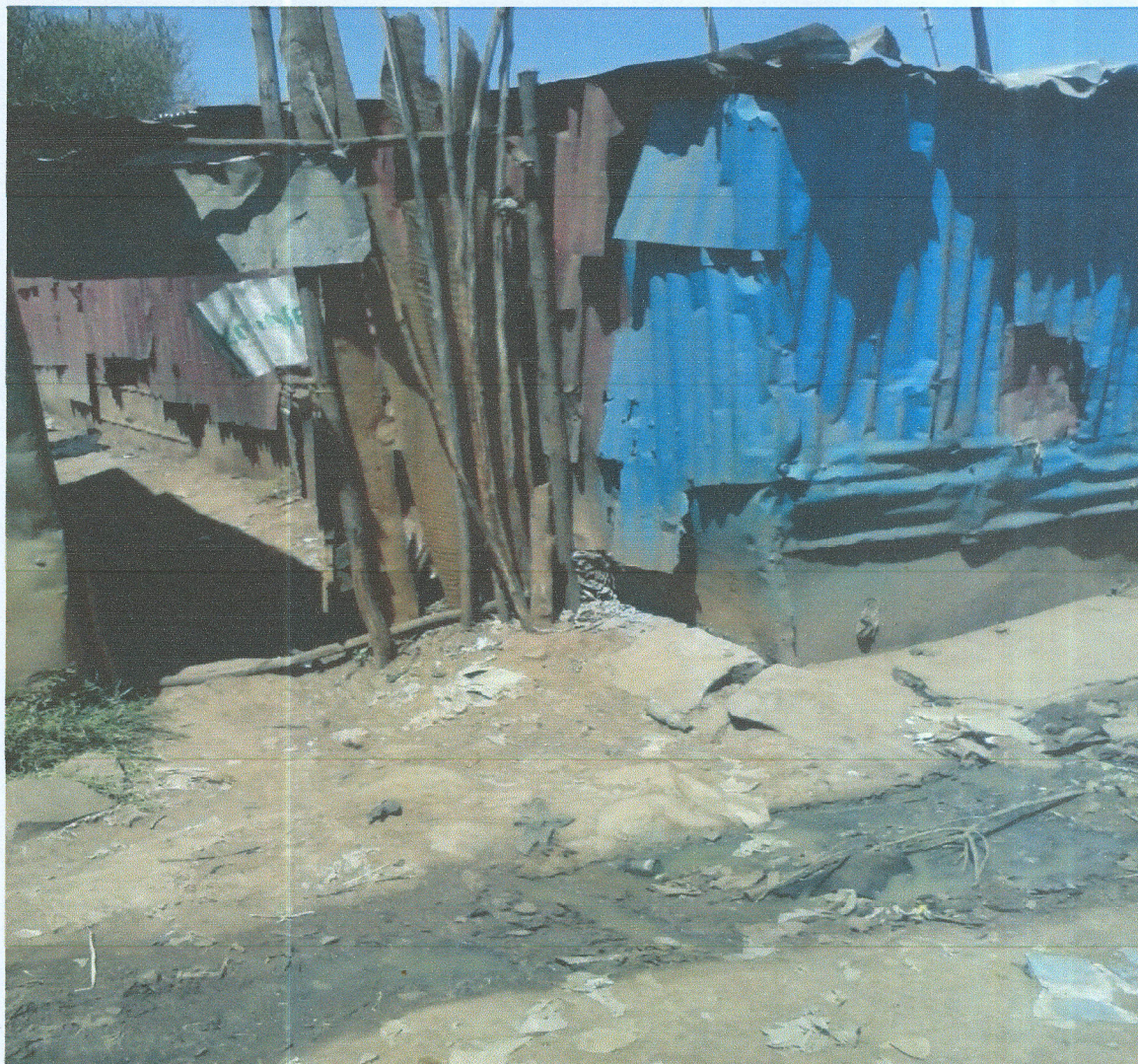
Figure 4.6a: Photograph showing poor drainage and shanty houses in Kiandutu slum
