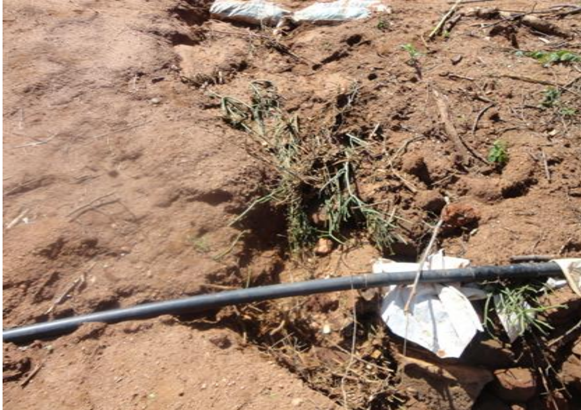
Plate 11: Pipes along Ndoo pipeline
