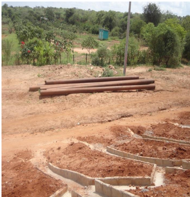
Plate 2: Replacement pipes used by TANATHI
