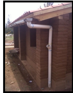
Figure 7. Rainwater catchment system
