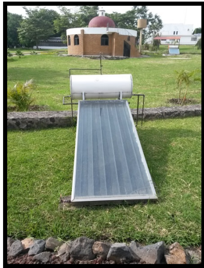
Figure 4. Solar water heater
