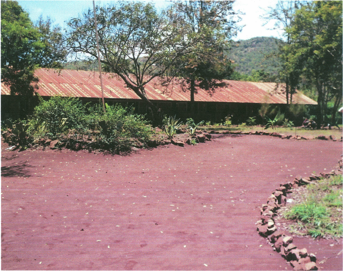
Plate 4.5 Rurii Primary School roof catchment with no water harvesting infrastructure in October 2012
