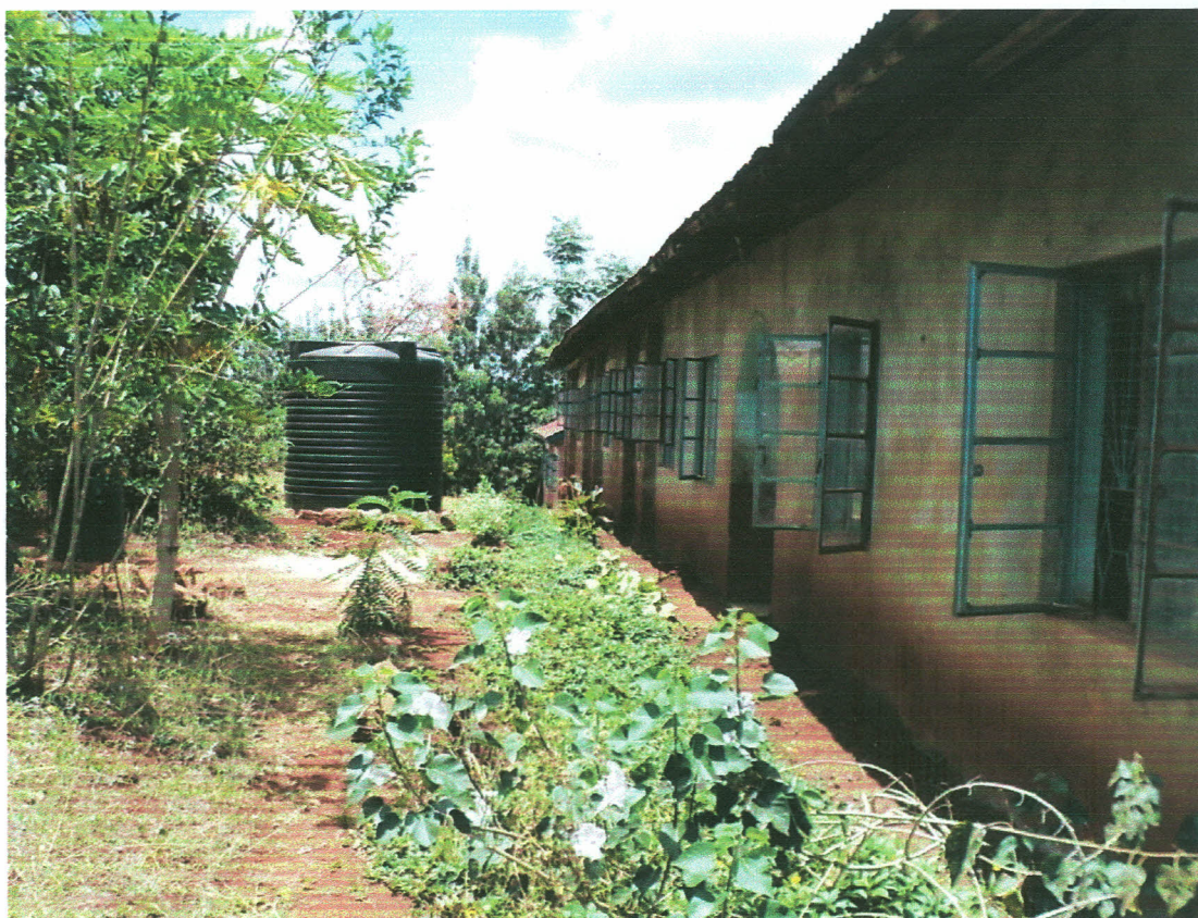
Plate 4.7 Muchungucha Primary School roof without gutters and an empty water storage tank donated by Safaricom in May 2012
