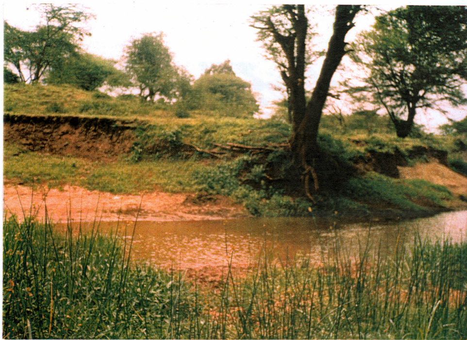
9: The banks of river Yanguni are heavily eroded and tree roots exposed. The river has vegetation growing on its bed thus reducing it to a puddle.
