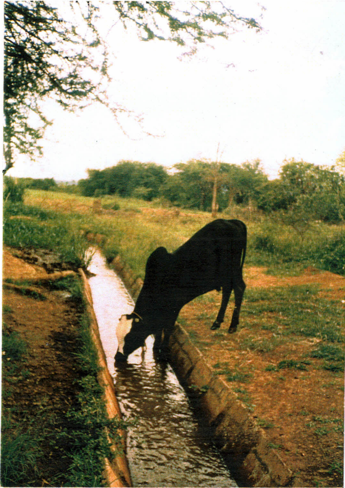
Plate 11: A cow drinking directly from the Ndalani canal. The slabs on the left side of the canal are loose due to erosion caused by animals gaining access to water. On the same side of the canal animal dung can be seen.
