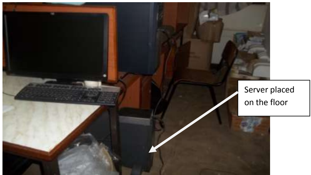
Plate 4.11: Server room which doubled as a store where server was placed on the floor. Source: Observation.
