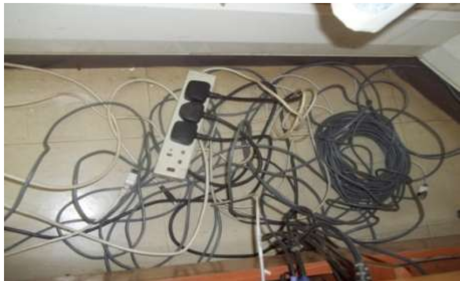
Plate 4.9: Power cables, network cables and multi plug all placed recklessly on the floor. Source: Observation.
