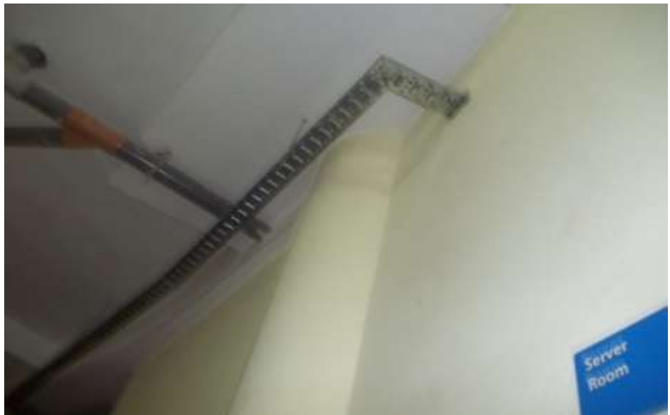
Plate 4.14: Server room located in the basement in one of the library buildings
