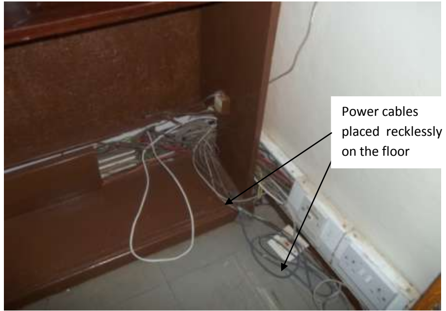
Plate 4.8: Power cables and network cables placed recklessly on the floor. Source: Observation.
