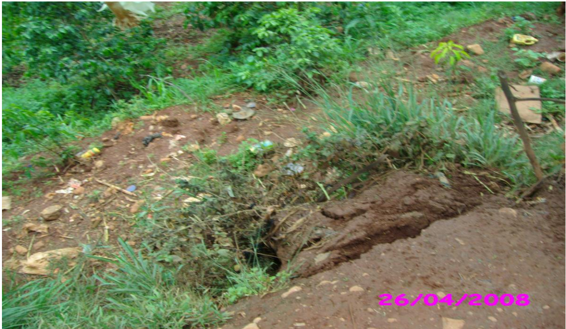
Plate 4.5: A landslide at Muooni dam site
