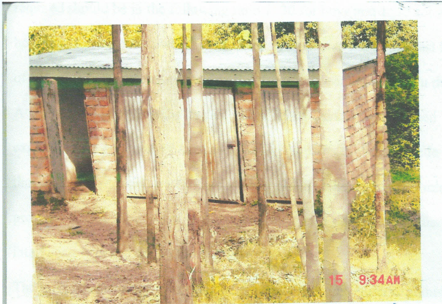
Figure 4.1: The state of toilets in a participating school
