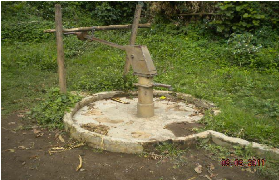
Plate 4.5: A dysfunctional borehole in Nyakinama Sub-county
