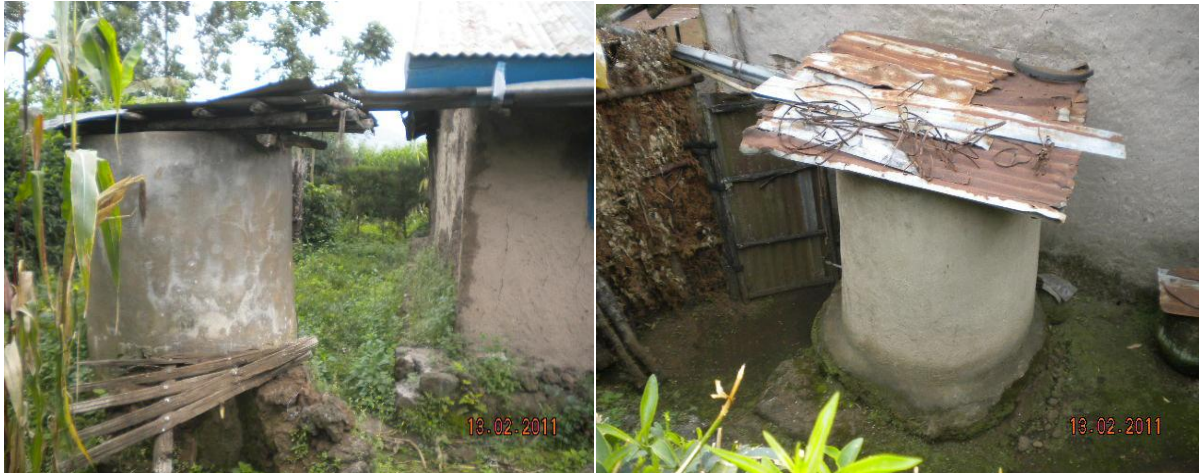
Plate 4.10: Example of Ferrocement Tanks in the sub-catchment (13/2/2011)
