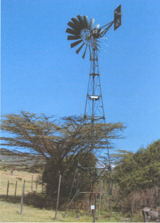
Plate 4-2: Borehole using wind energy at Aitong town centre. (Source: Author, 30/8/2012)
