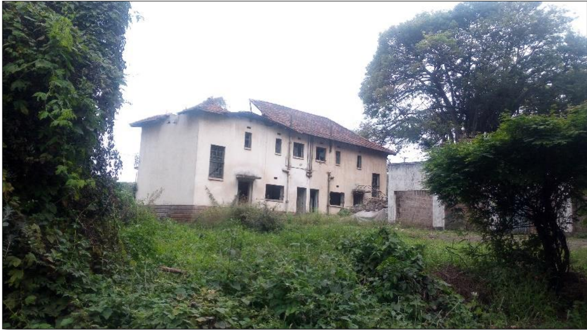
a) Dilapidated buildings low rise building along Third Avenue, Ngong road
