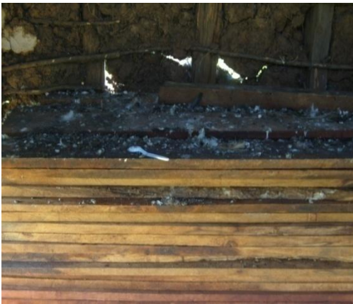
Plate 3: Chicken droppings on top of timber inside an abandoned house.
