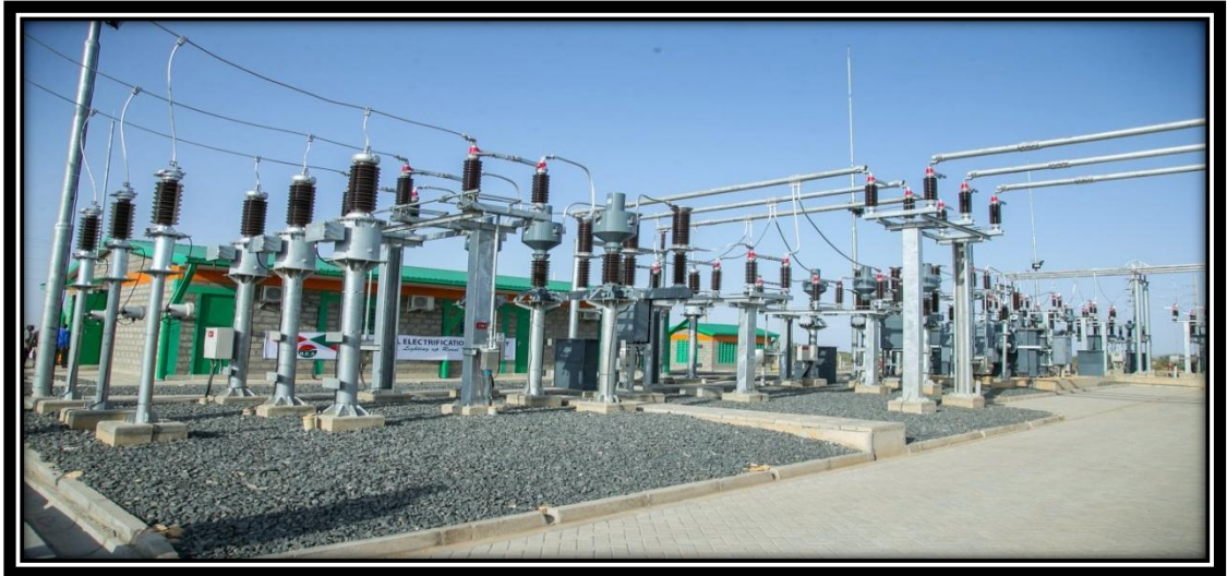
Plate 4.20: The Lokichar substation electricity project
