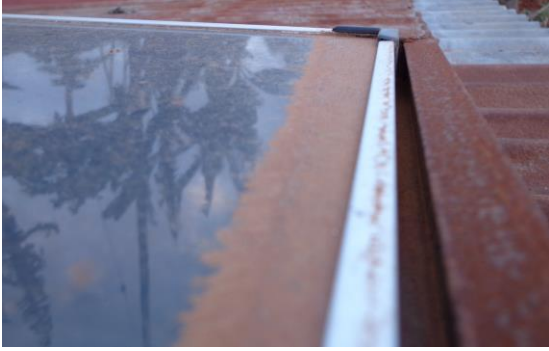
Figure 5.6: 18W amorphous module type showing a portion of cells covered by a thick layer of dust
