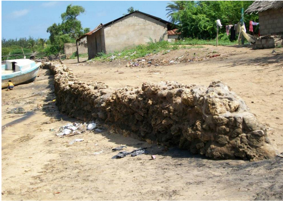
Photo 4.3: Construction of a sea/stone wall at Ngomeni village in Malindi. (Photo by B. Akunga).
