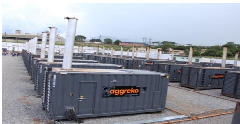
Fig. 7. Diesel generators in operation in Malawi
