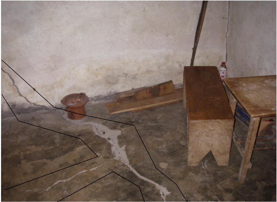
Plate 6.2b: A cracked house floor Sironko (August 2009)
