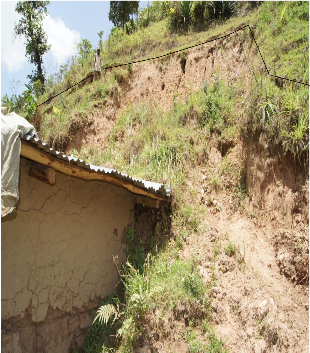
Plate 4.10: Slope failure triggered by undercutting by housing construction (Maboono July 2010)
