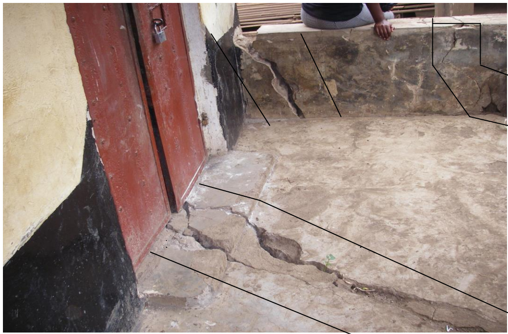
Plate 6.2a: A cracked house veranda (Kibooko-August2009)
