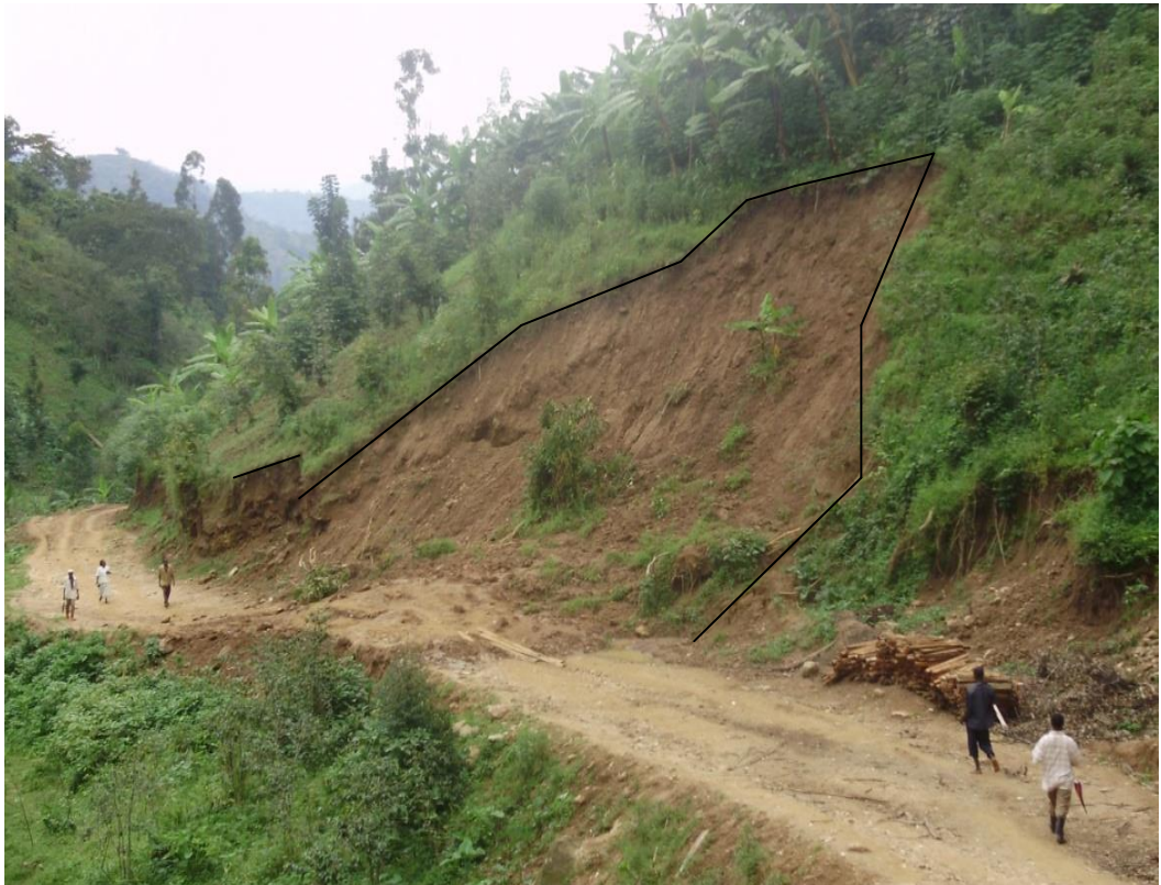
Plate 4.9: Slope failure experienced along Bukhalasi-Namesti road on 4 th March 2010 (Bukhalasi 23 rd March 2010)
