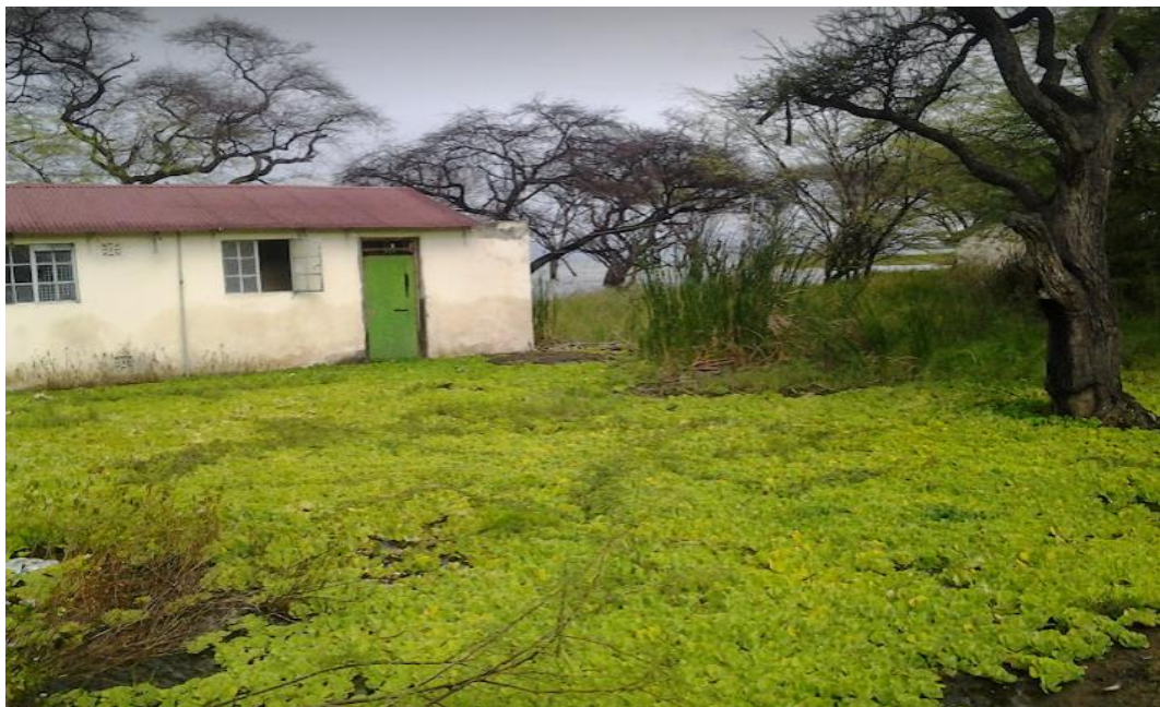
Flooded and abandoned schools and offices following flooding of Lake Baringo in 2012
