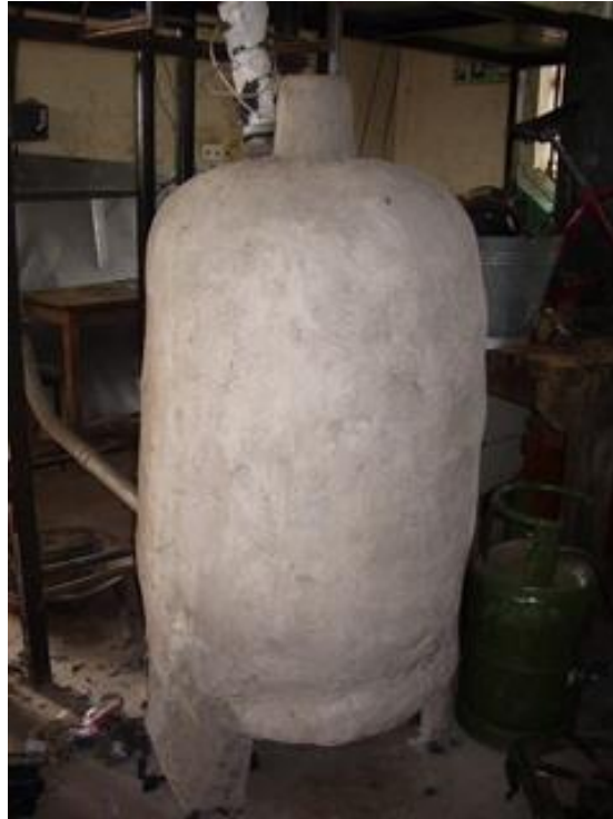
Figure 3.11 Complete boiler –storage system with a layer of Plaster of Paris above woollen blanket insulation
