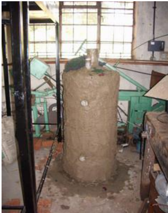
Figure 3.9 Boiler insulated with a layer of vermiculite
