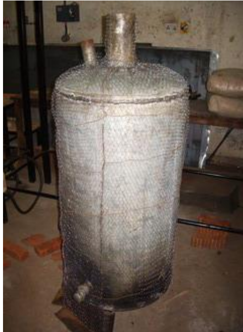
Figure 3.8 An un-insulated boiler covered with a layer of chicken wire
