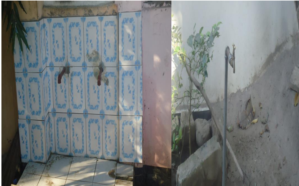
Plate 4.4: Household Stand Pipes type of Kiosk at Tabata Area of Msimbazi sub catchment ( Field Survey, 2012 )
