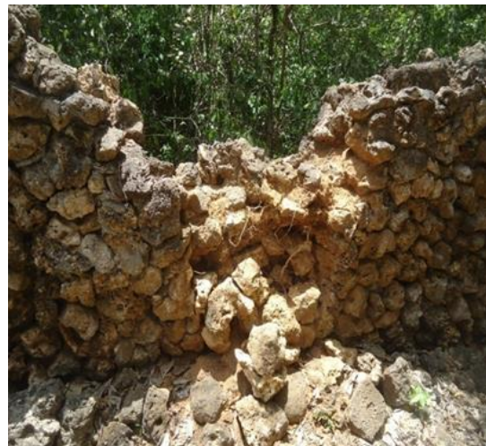
Plate 3.6: Part of the inner wall that is disintegrating due to the effect of tree roots burrowing into the wall Source: NMK Gedi
