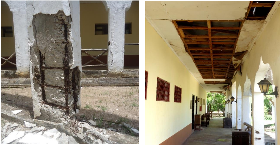
Pate 2.9: The wooden balustrade along the circular walkway is disintegrated due to the effects of wet and dry
