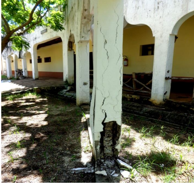
Plate 2.8: Showing pillars that have decayed
