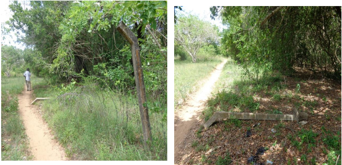
Plate 3.12: Part of the fence at the site with broken concrete pillars
