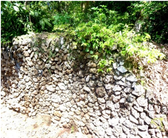
Plate 3.2: Vegetation Growth on Walls of monuments
