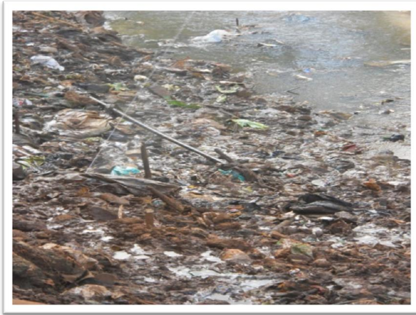
Plate 5.4: Leaking Water Pipe beside a Sewer
