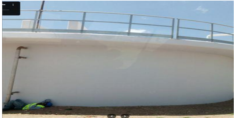
Water treatment system at Konza Konza Technopolis, 2024
