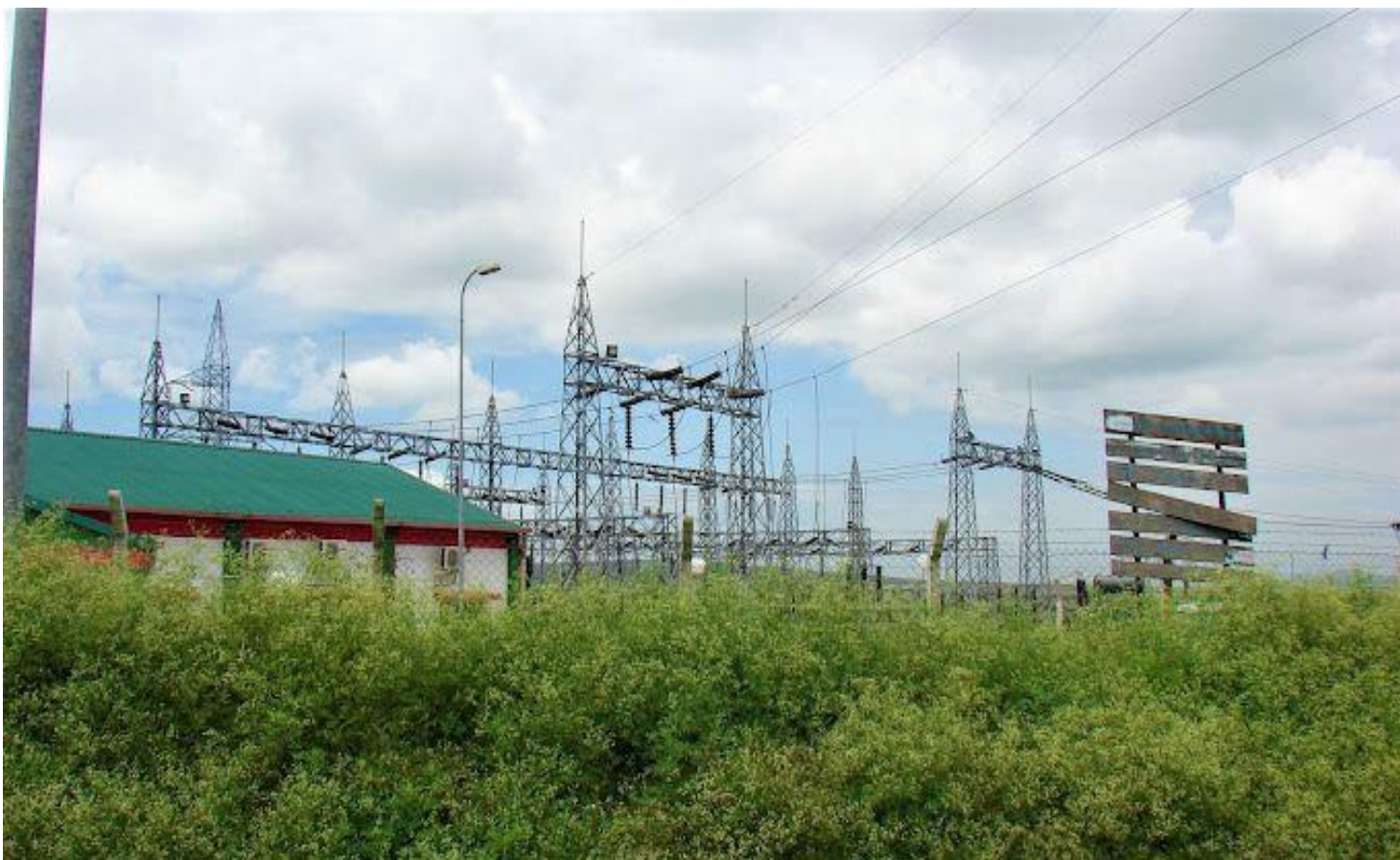
KETRACO Konza Substation. Google Maps, 2023
