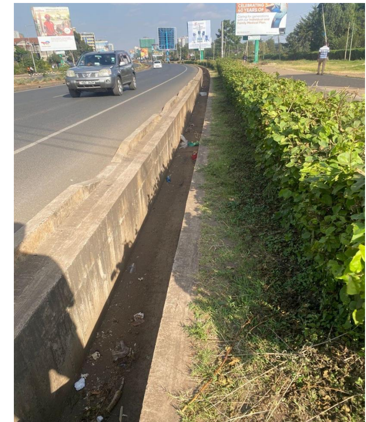
View the open drainage along Ngong Rd. Source: Authors, 2025
