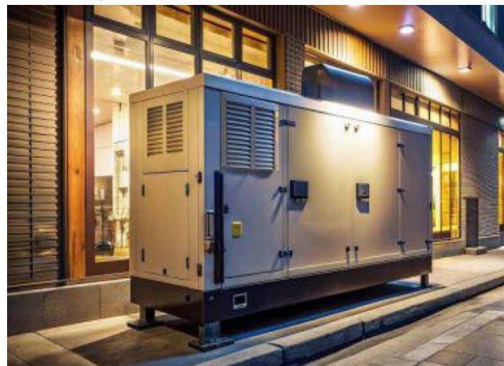
Backup generator Source: Generators Direct
