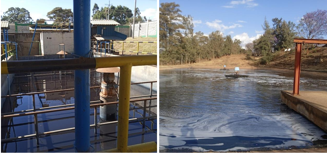
An effluent treatment plant for liquid waste
