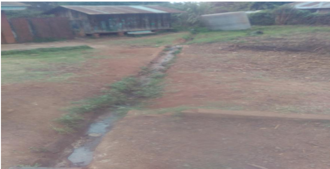
Figure 4.11: An Example of a Dirty, Open Drainage Channel to Dispose Waste Water from a Dining Hall
