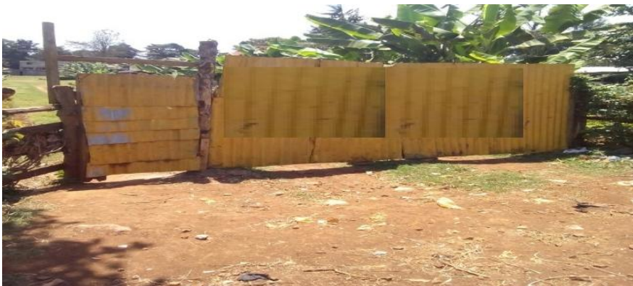
Figure 4.12: An Example of a Poorly Constructed and Insecure School Gate
