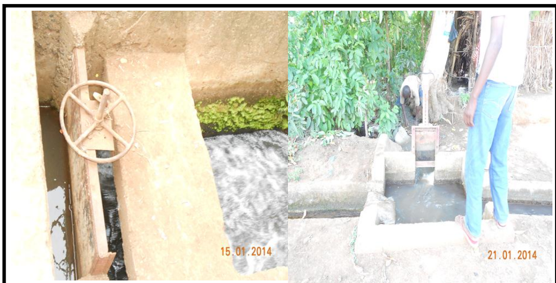
Plate 4.11: Intake gates for water allocation in Kiladeda (Source: Author, 2014)
