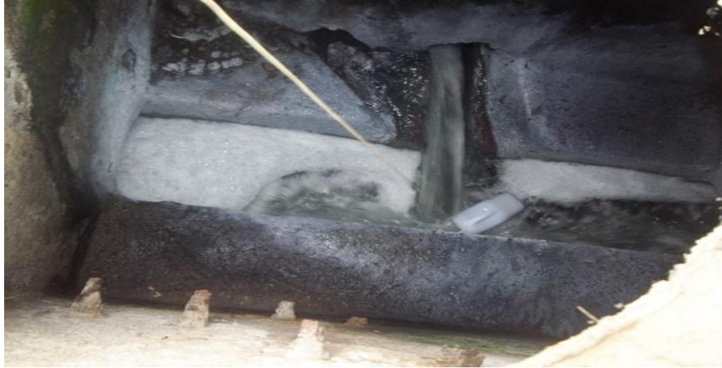
Plate 3. 6: Effluent flow through the municipal sewer. 7 th August 2013 at 10 a.m.
