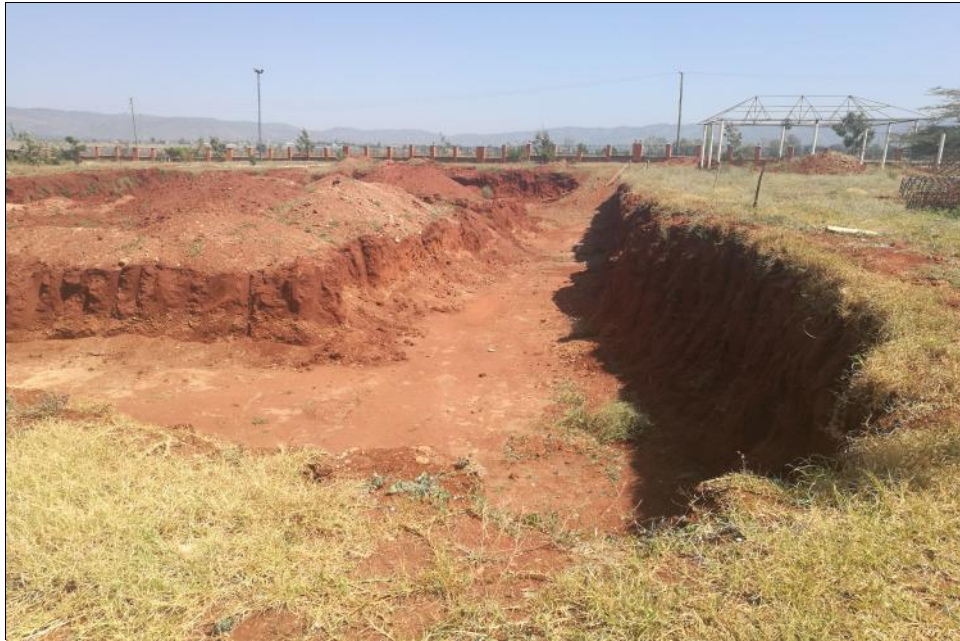
Plate 4.16: Unsecured ditch in the park
