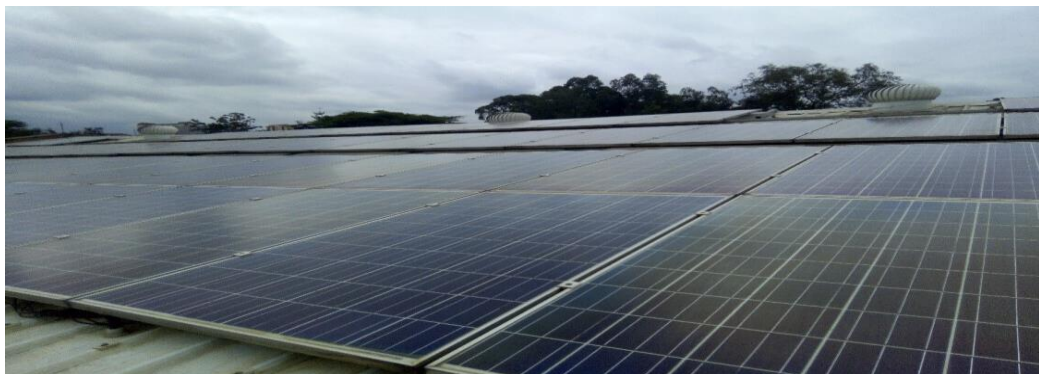
Figure 3.3: Grid connected solar Photovoltaic system at Strathmore Energy Research Centre building
