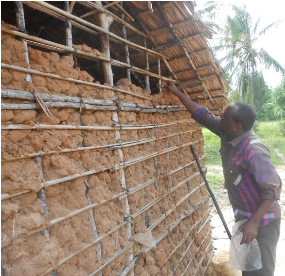
Appendix 3: Wall sample being collected from a typical mud wall of a hut in the Mrima hill region
