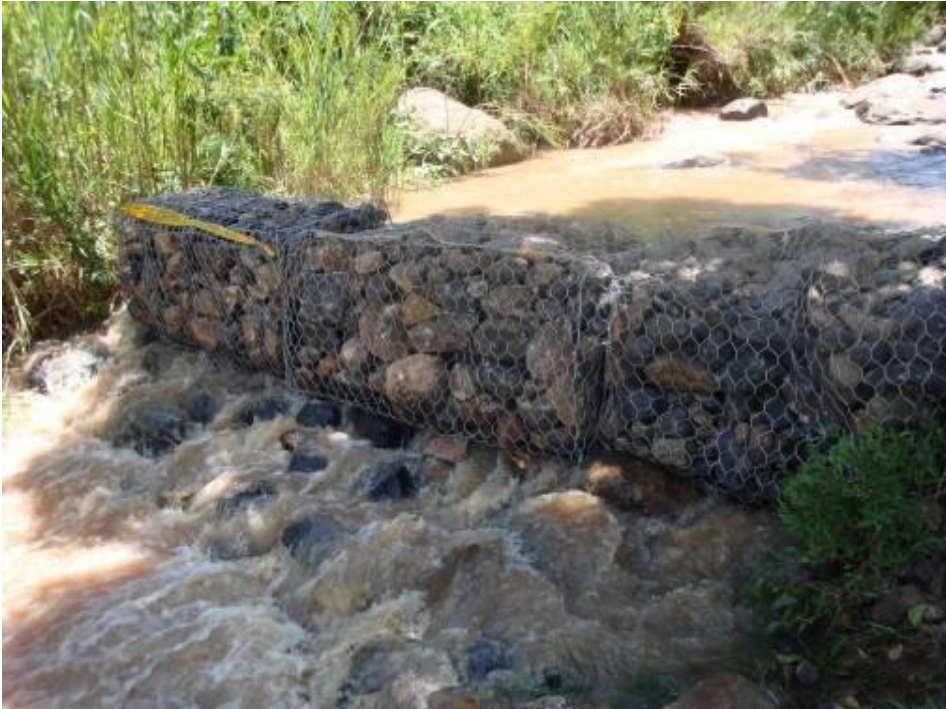
Plate 7. Gabion weir constructed at Mid-stream Kisian River (site KS2), following the breakdown of boulder weirs.
